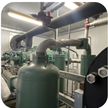
NH 3 refrigeration system - Plastuni Operations
