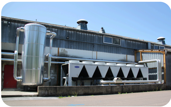
Heat recovery system
