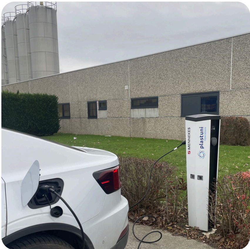
Electric vehicle charging stations - Plastuni Operations
