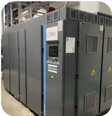
New compressor - ANL Wellen
